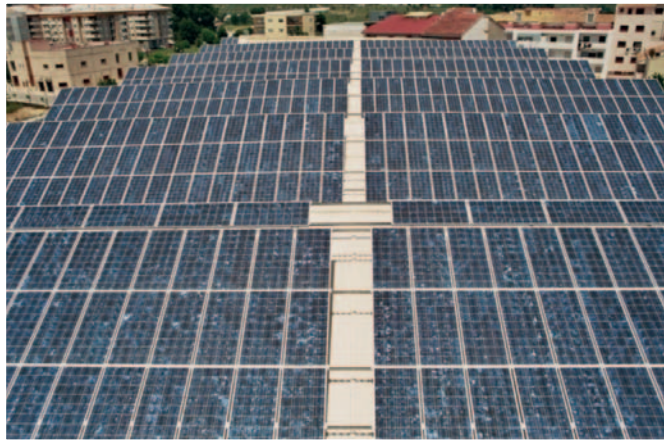
100 kW Solar Power Plant (Alicante)
