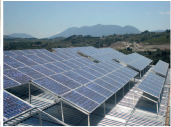
100 kW Solar Power Plant (Alicante)
