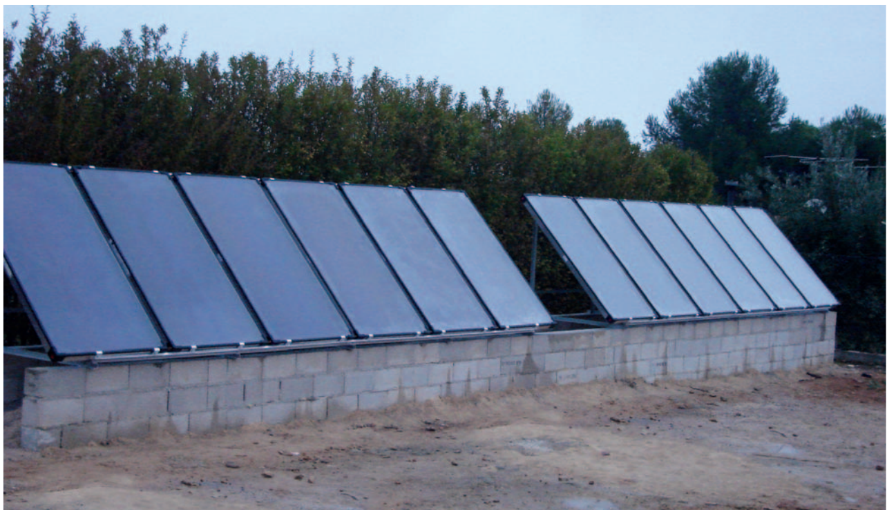
Solar water heating for domestic hot water and underfloor heating in a house in Cocentaina (Spain).
