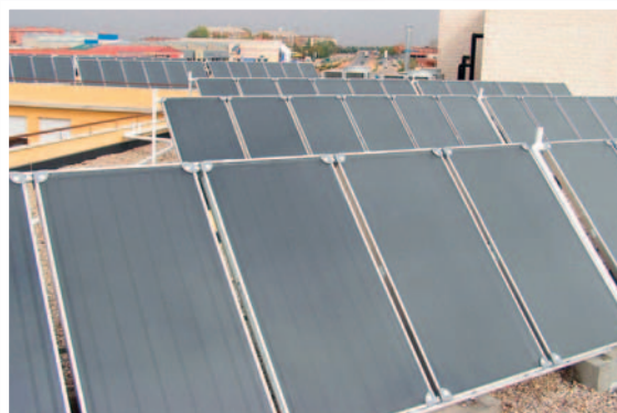
Solar water heating in a hotel.
